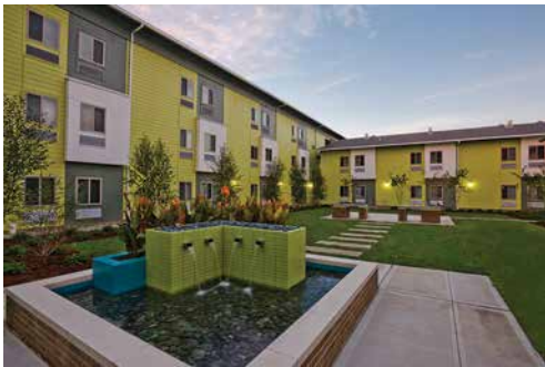
Multi-family housing has extruded aluminum trim above windows and doors, between fiber cement siding and brick, and on inside corners.
