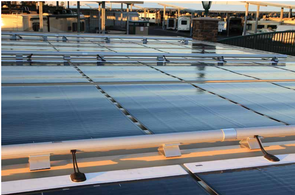
Figure 1 Solar power systems can help commercial buildings and residential home owners avoid the unexpected fluctuations in energy prices as well as help reduce carbon emissions from fossil fuel power sources.
