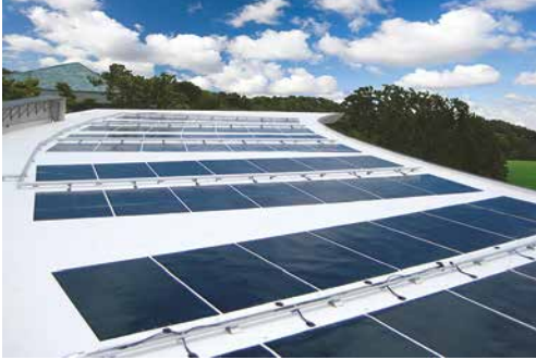
Figure 4 Flexible and flat, modern solar modules can help increase overall solar collection capacity while not interfering with the roof aesthetics.
